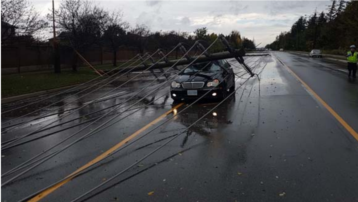
Figure N01 - 11: Pole failure due to Microburst on October 15, 2017
